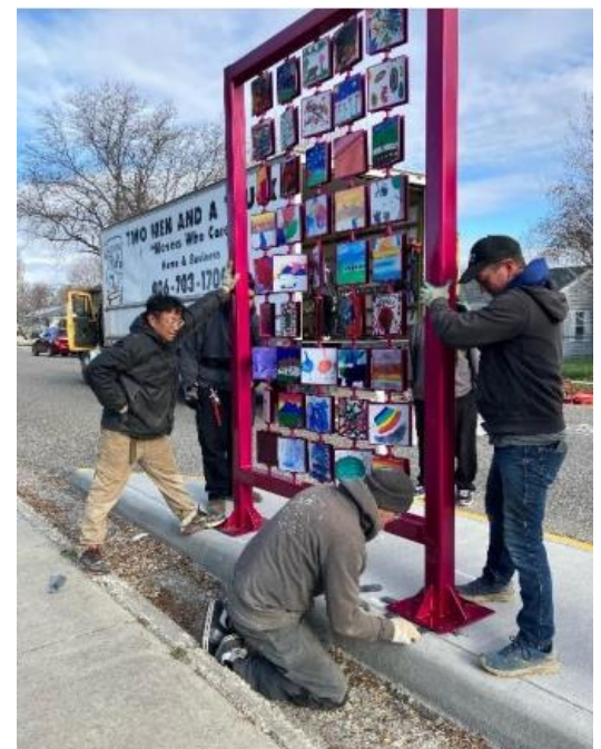
Installation of Terri Porta's and McKinley Elementary students' sculpture at the intersection of 10 th Ave. N and Ave C.
