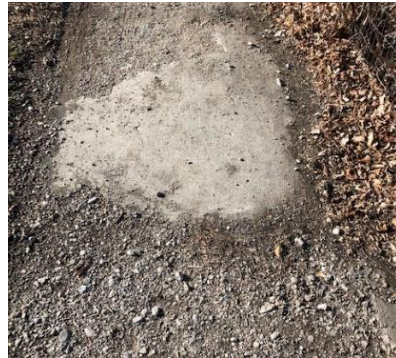
Other unsafe conditions
