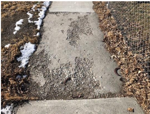
Rough, chipped surface
